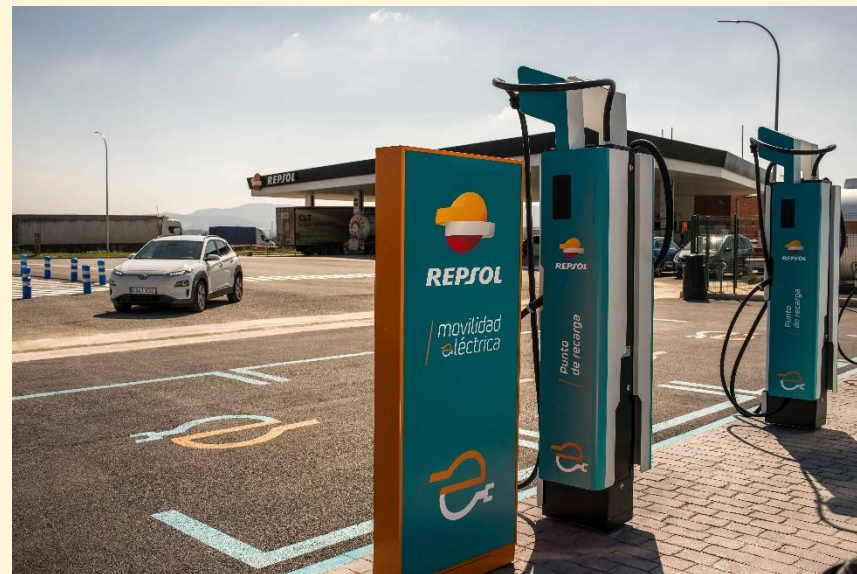
Photo: Repsol electric charging points in Spain and Portugal
